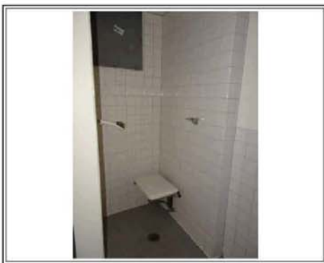
MEN'S RESTROOM IN THE BASEMENT
