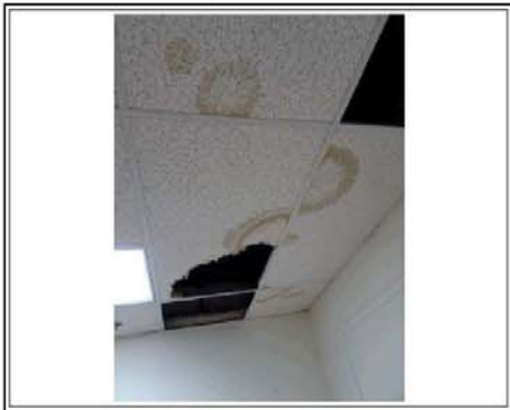
EXAMPLE OF WATER DAMAGE IN THE CEILING OF THE FIRST FLOOR
