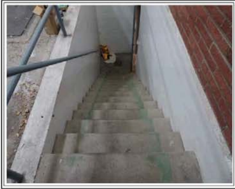
STAIRS FROM THE GARAGE AREA OF THE FIRST FLOOR TO THE BASEMENT
