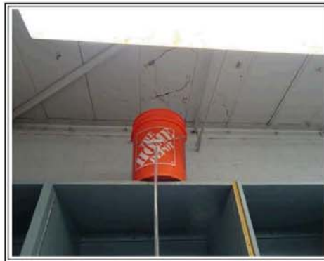
BUCKET USED TO PREVIOUSLY CATCH WATER FROM LEAKS IN THE CEILING
