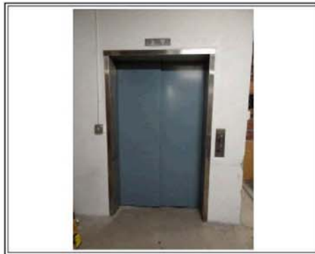
ELEVATOR IN THE GARAGE AREA OF THE FIRST FLOOR
