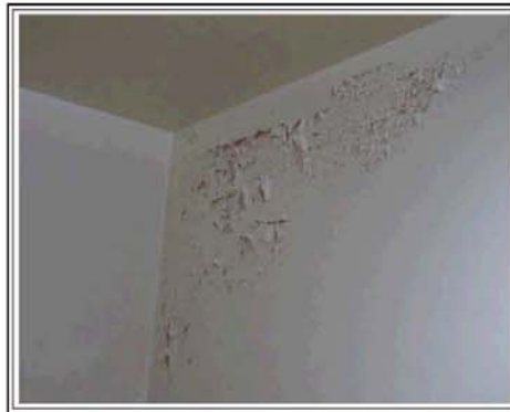
EXAMPLE OF WATER DAMAGE IN THE WALL OF THE UNISEX RESTROOM ON THE FIRST FLOOR
