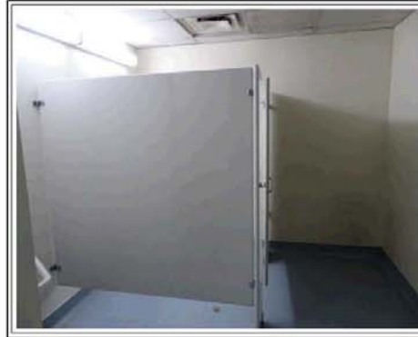
MEN'S RESTROOM IN THE BASEMENT
