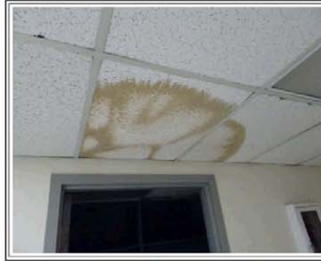
EXAMPLE OF WATER DAMAGE IN THE BASEMENT CEILING
