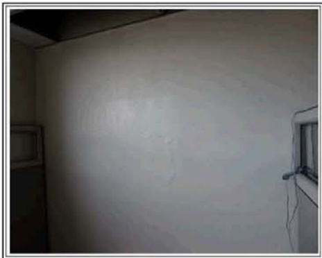
EXAMPLE OF WATER DAMAGE ON AN EXTERIOR WALL ON THE FIRST FLOOR
