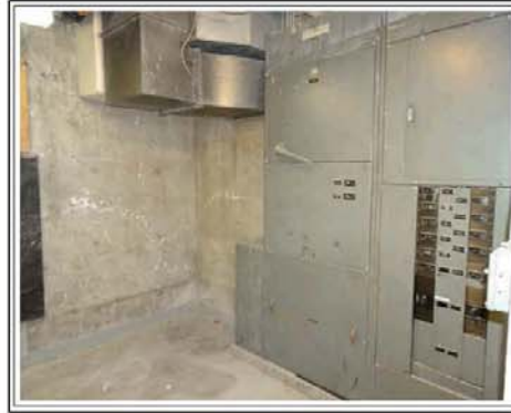
MECHANICAL ROOM IN THE BASEMENT
