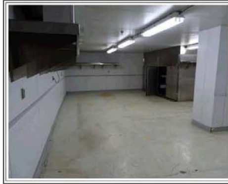
COLD ROOM IN THE BASEMENT
