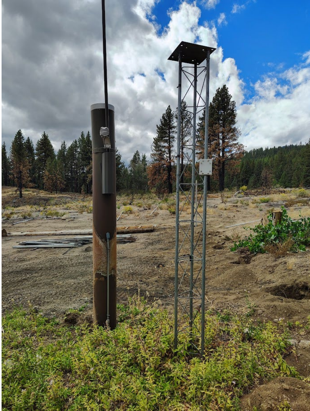
Example of a Rohn tower (on right) at the former Davis Creek Park station. The proposed tower will be several feet shorter.
