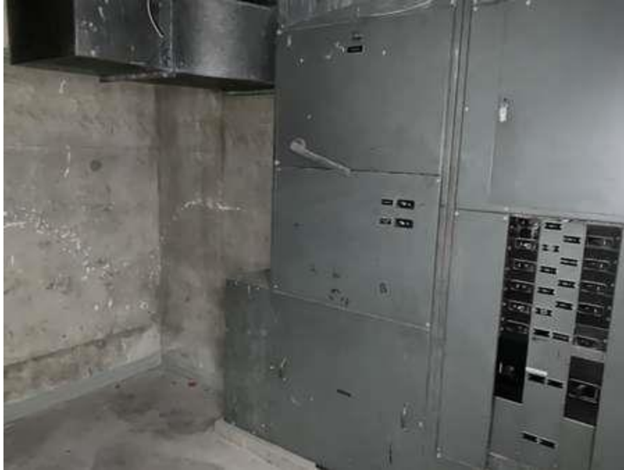
Subject Basement – Service Panel
