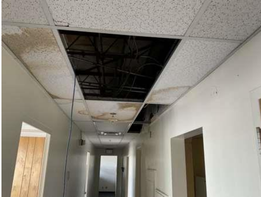
Subject Interior Dropped Ceiling Panels and Staining
