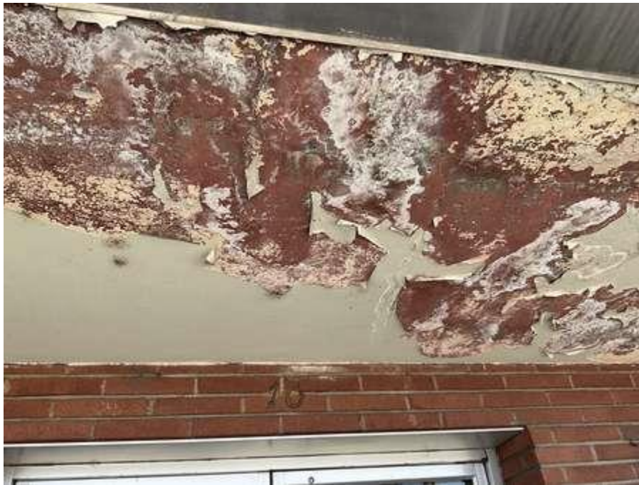
Underside of Porch Ceiling (Deferred Maintenance)
