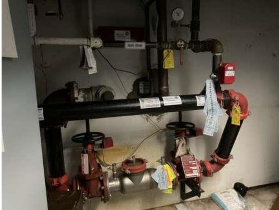
Subject Fire Sprinkler System Main
