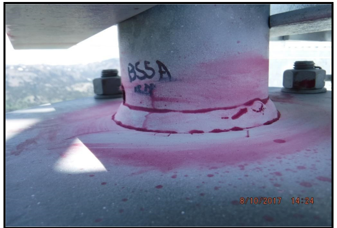
Center Bead Cracking Typical
