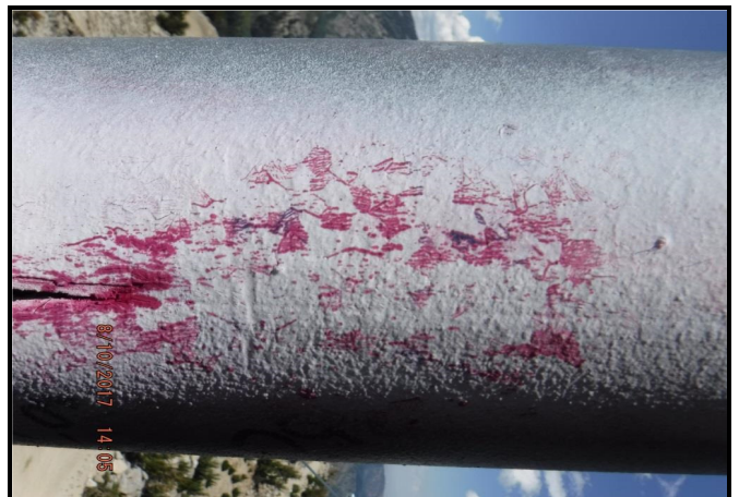
Cracking above Split
