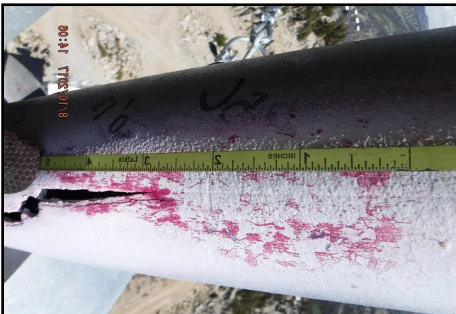
Cracking 3" above Split
