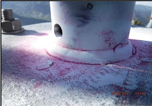
Flange with No Indications
