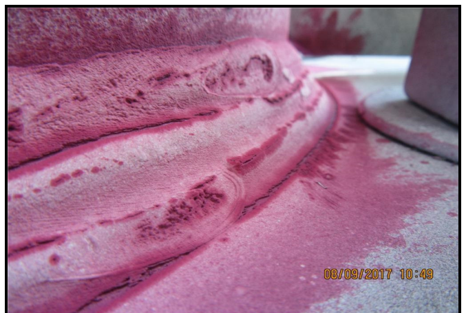
Base Flange Cracking
