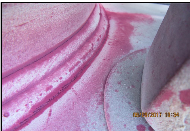
Base Flange Cracking
