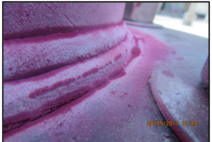
Base Flange Cracking
