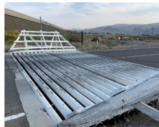
New Cattle Guard at Site Entrance
